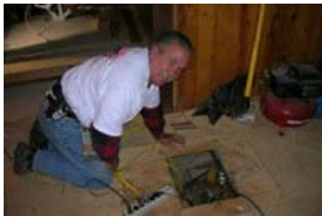
We found some unexpected work that needed to be done under the bedroom floor. Here Manny Rebello is talking to the "tunnel rats" that volunteered for this mission.
