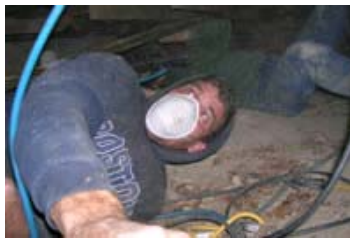
And the tunnel rats were (front) Phil Roos owner of Preferred Construction and (background) brother John Roos owner of Roos Construction. Nice work guys!!
