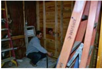
Progressive Plumbing and Piping provided the plumbing expertise and really stepped up to the plate, crawling under the house and running the plumbing wherever it was needed!
