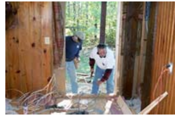
The kitchen was too small for wheelchair accessibility, so a "bump-out" was made for the refrigerator to make the needed room. Here Kirt Rebello and Manny Rebello "make a hole."
